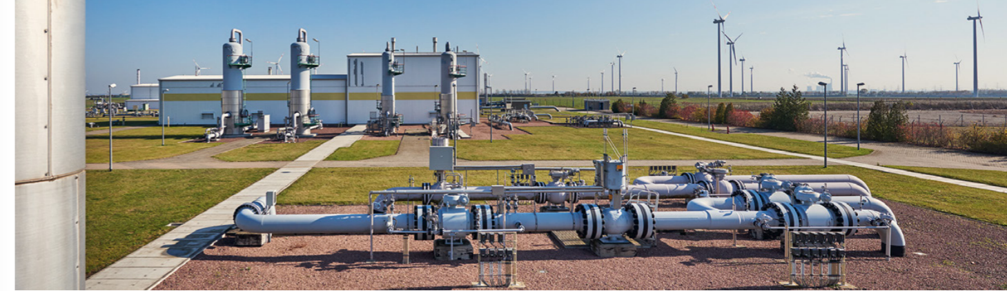
The cavern storage facility is one of the core elements of the Energy Park.
