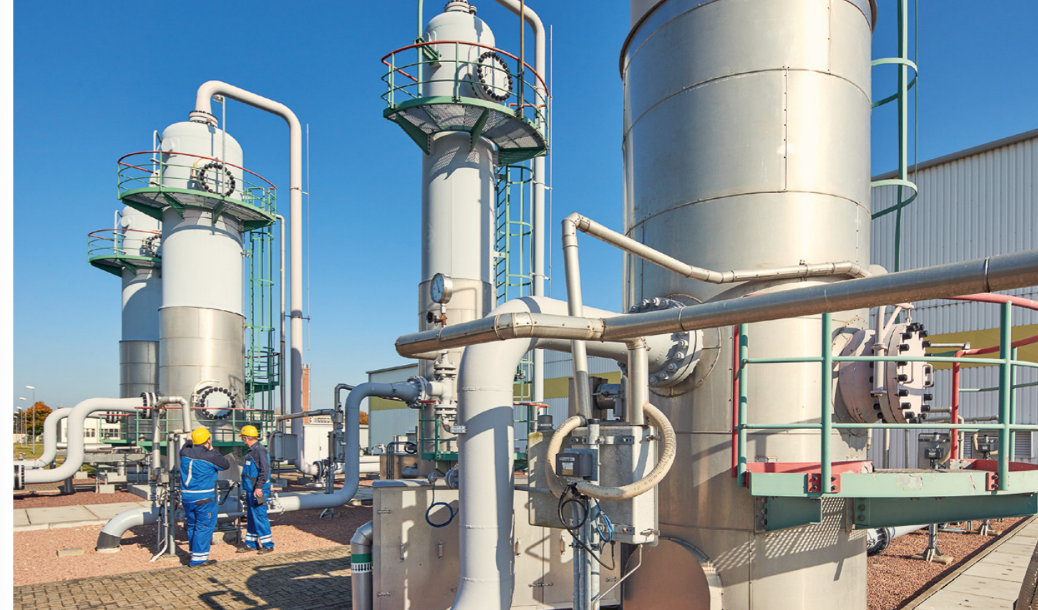
Cavern storage Bad Lauchstädt: Preparations for storing green hydrogen
