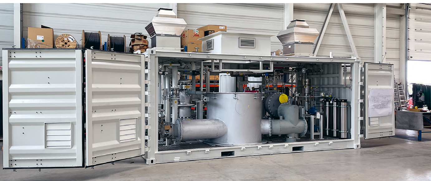
Plant for steam reforming of natural gas from the HydroGIn preliminary project for conversion to biogas operation in the BioHydroGen project.
